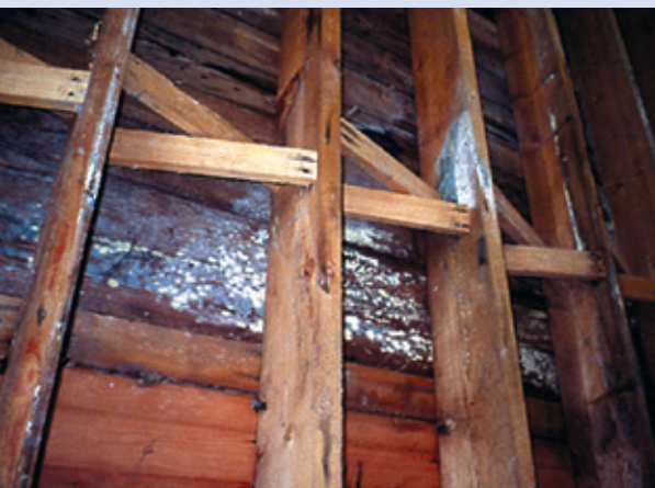
Photo 6: Heavy mold growth on underside of spruce floorboards
