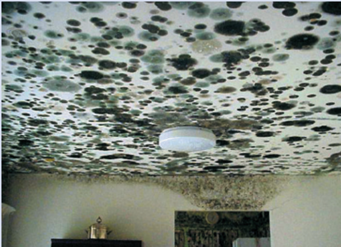
Photo 2: Extensive mold contamination of ceiling and walls
