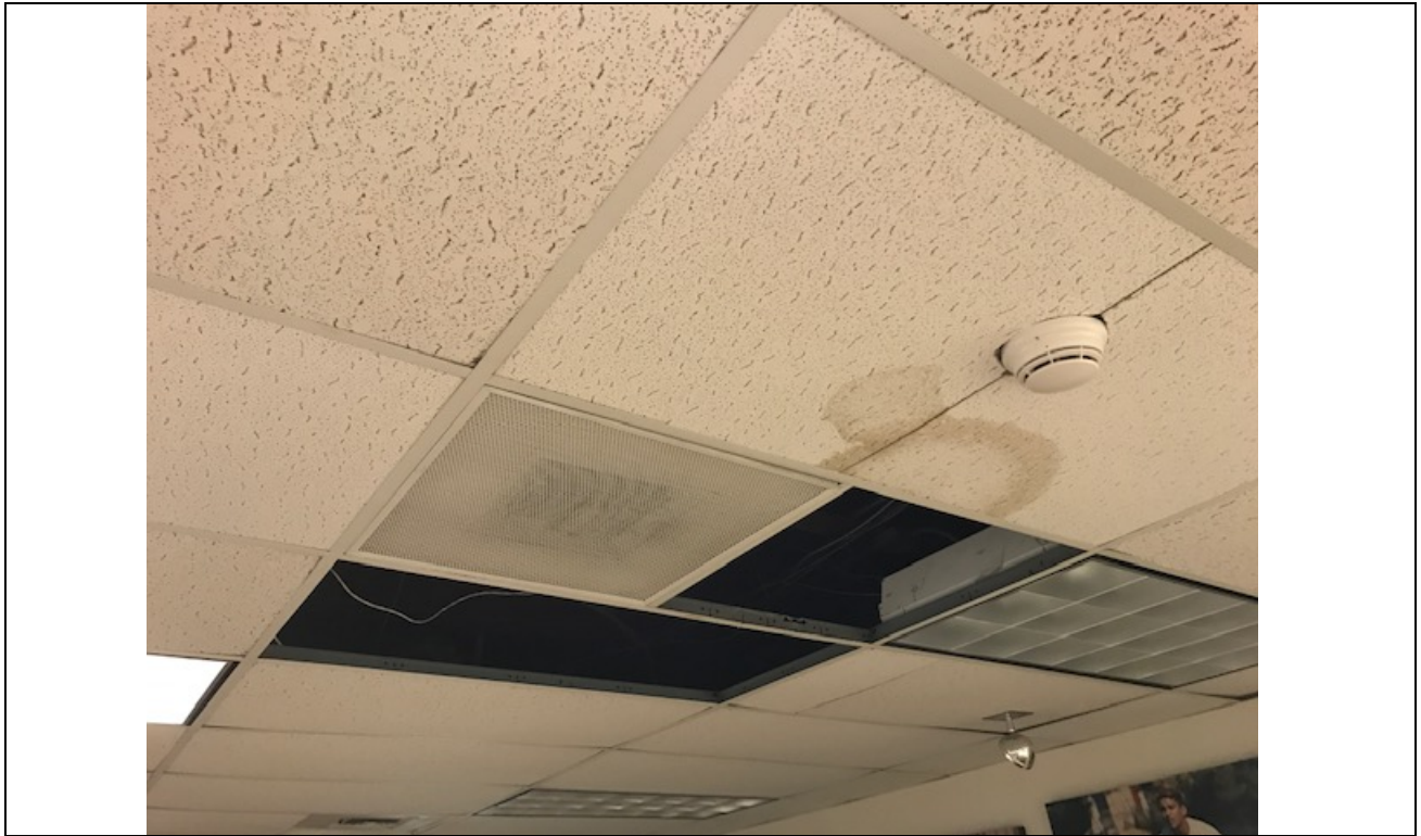
Photo No. 11: CB Building, Room 215 – Water-stained / missing ceiling tiles.
