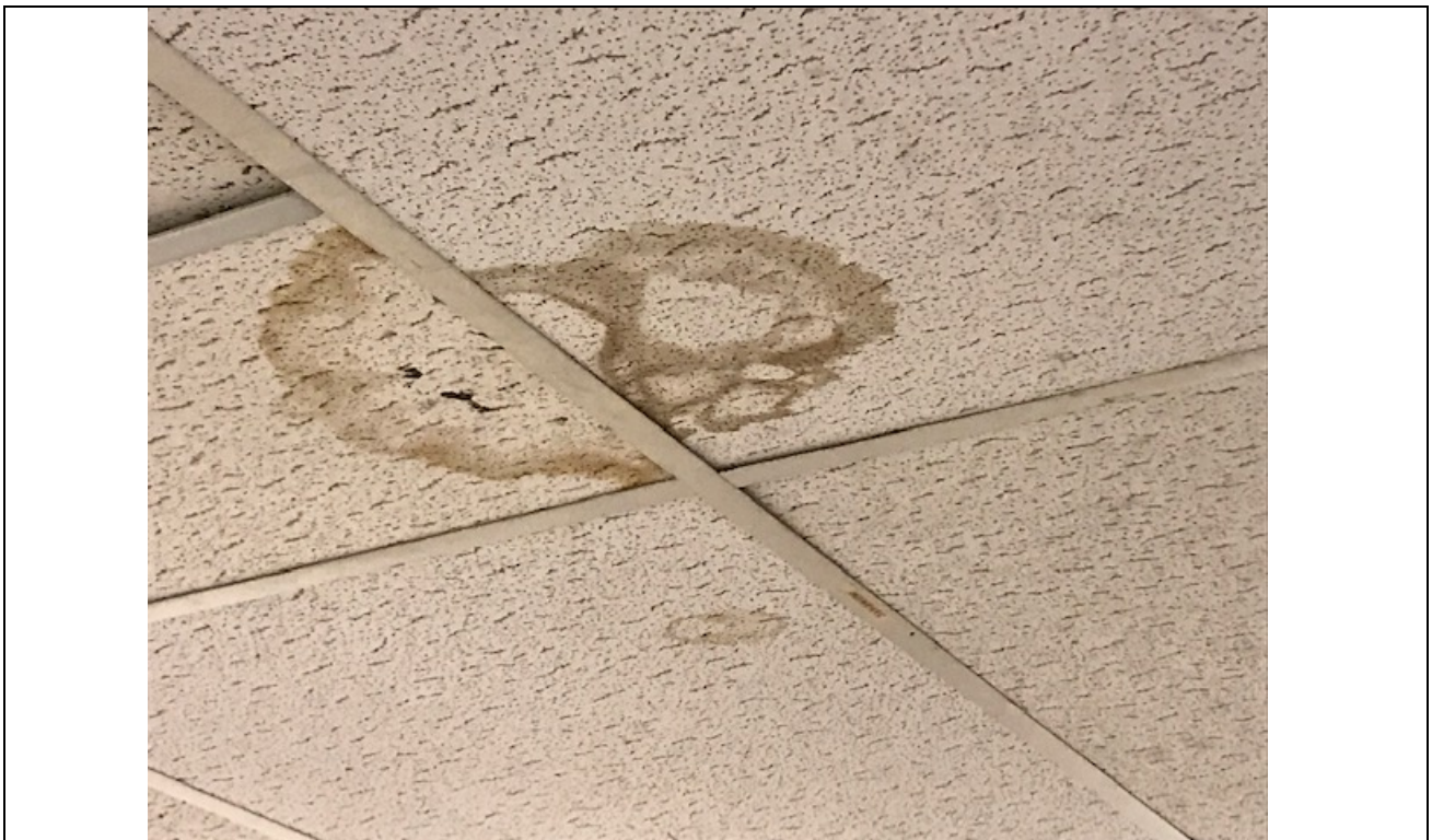
Photo No. 12: CB Building, Room 215 – Water-stained ceiling tiles.
