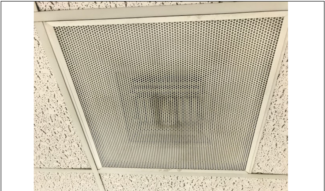
Photo No. 2: CB Building, Room 109 – particulate matter and accumulated dust on air supply diffuser.
