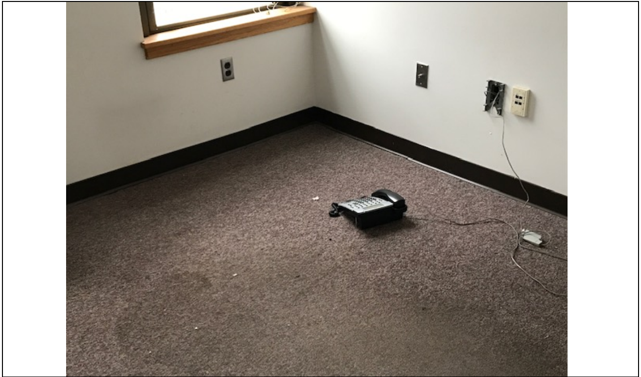
Photo No. 7: CB Building, Room 204 – Heavily-stained carpeting.
