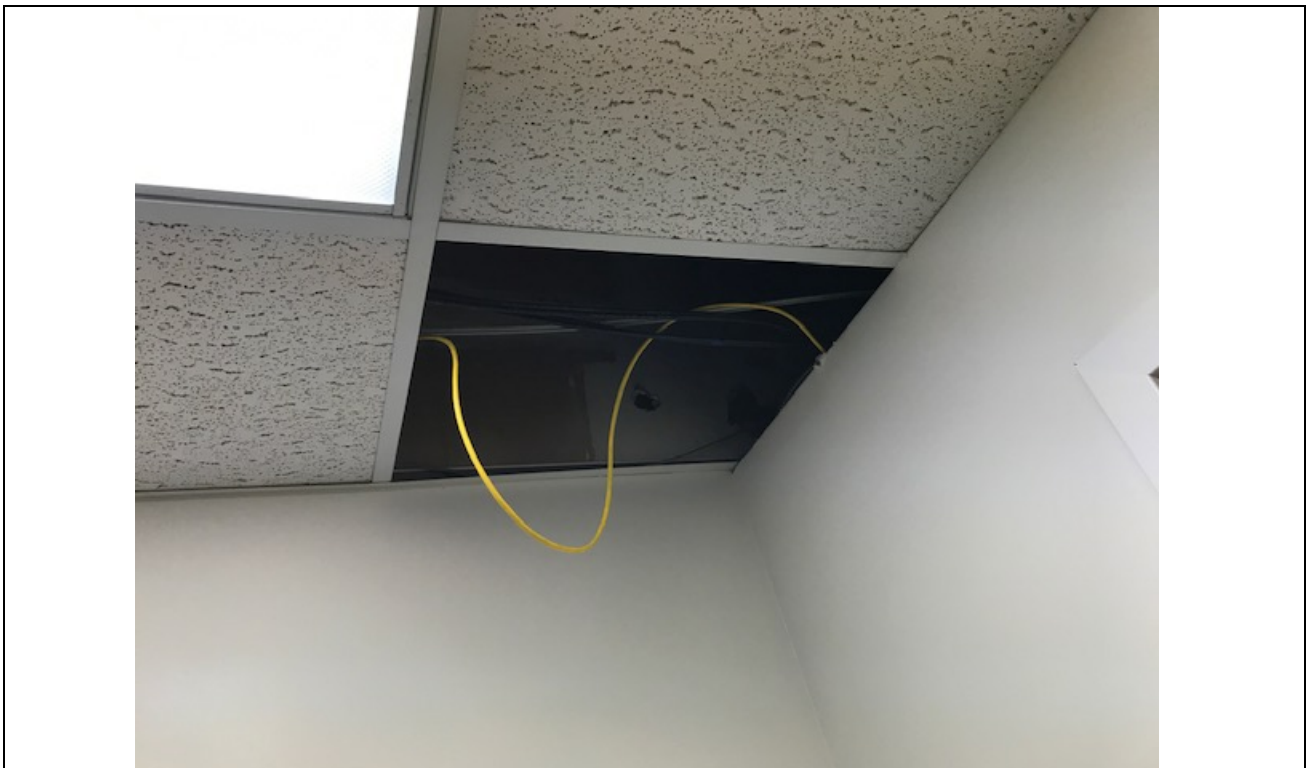
Photo No. 4: CB Building, Room 122 - Missing Ceiling Tile.
