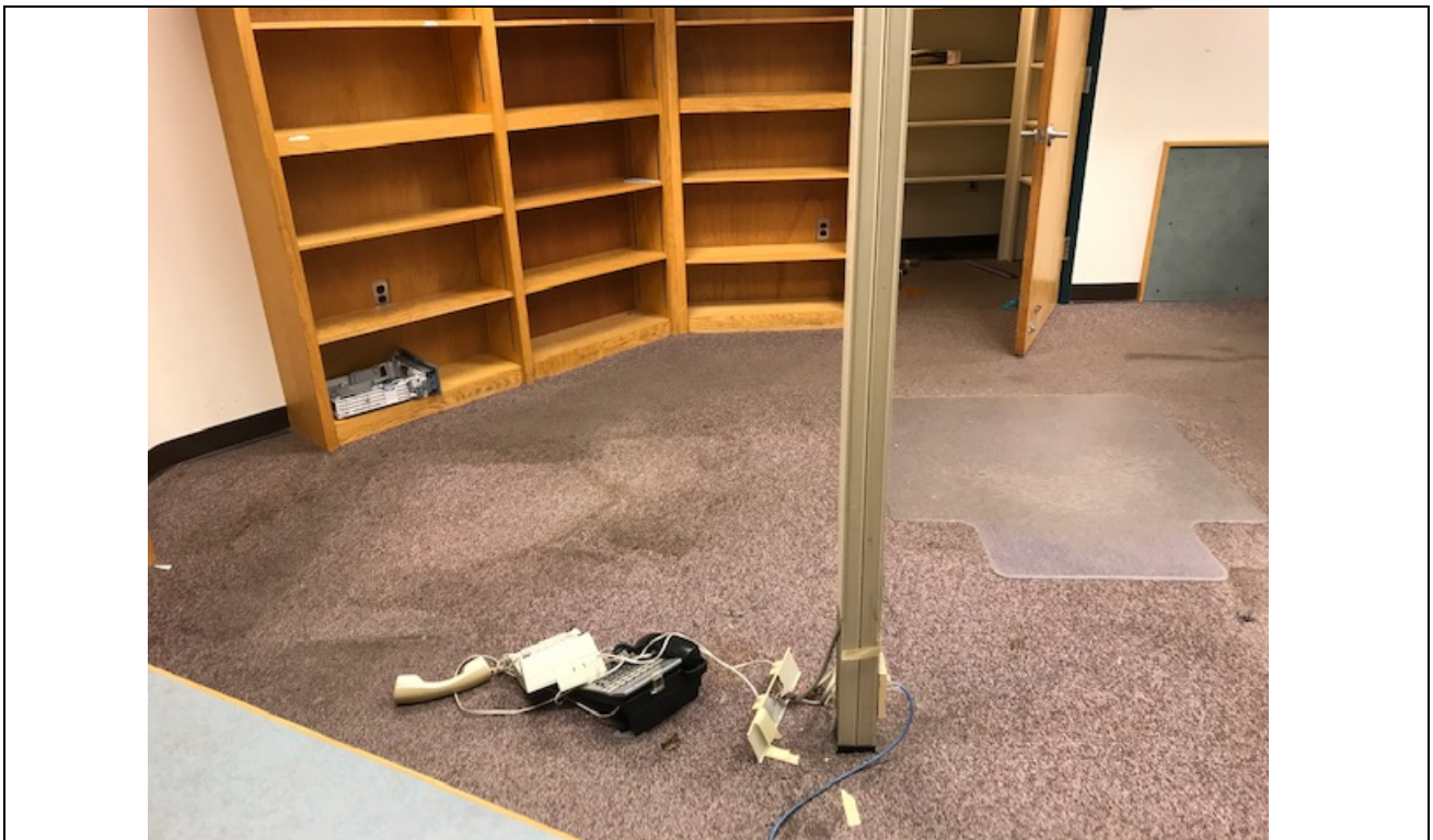
Photo No. 10: CB Building, Suite 215 (Center) – Heavily-stained carpeting.
