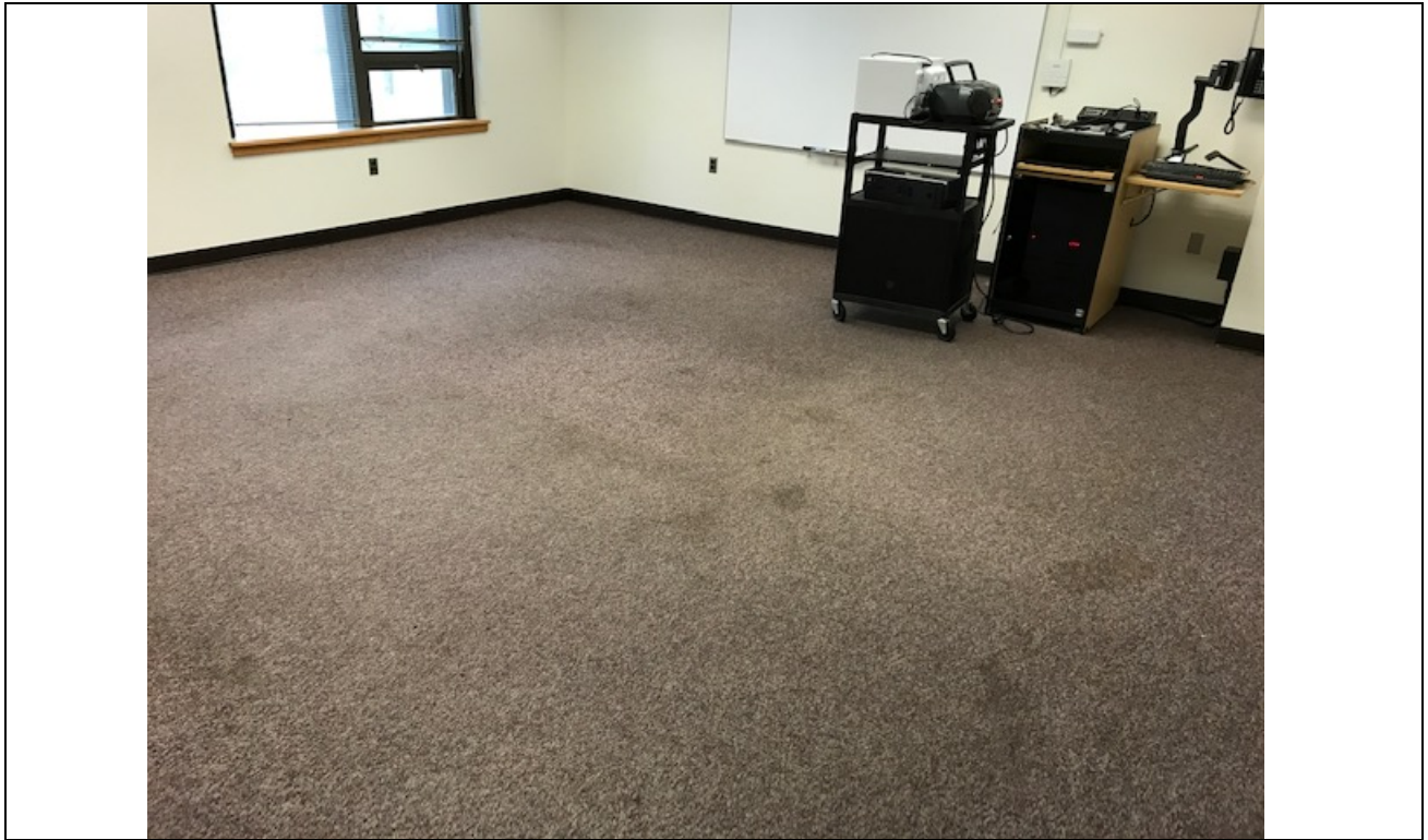
Photo No. 9: CB Building, Room 218 – Heavily-stained carpeting.
