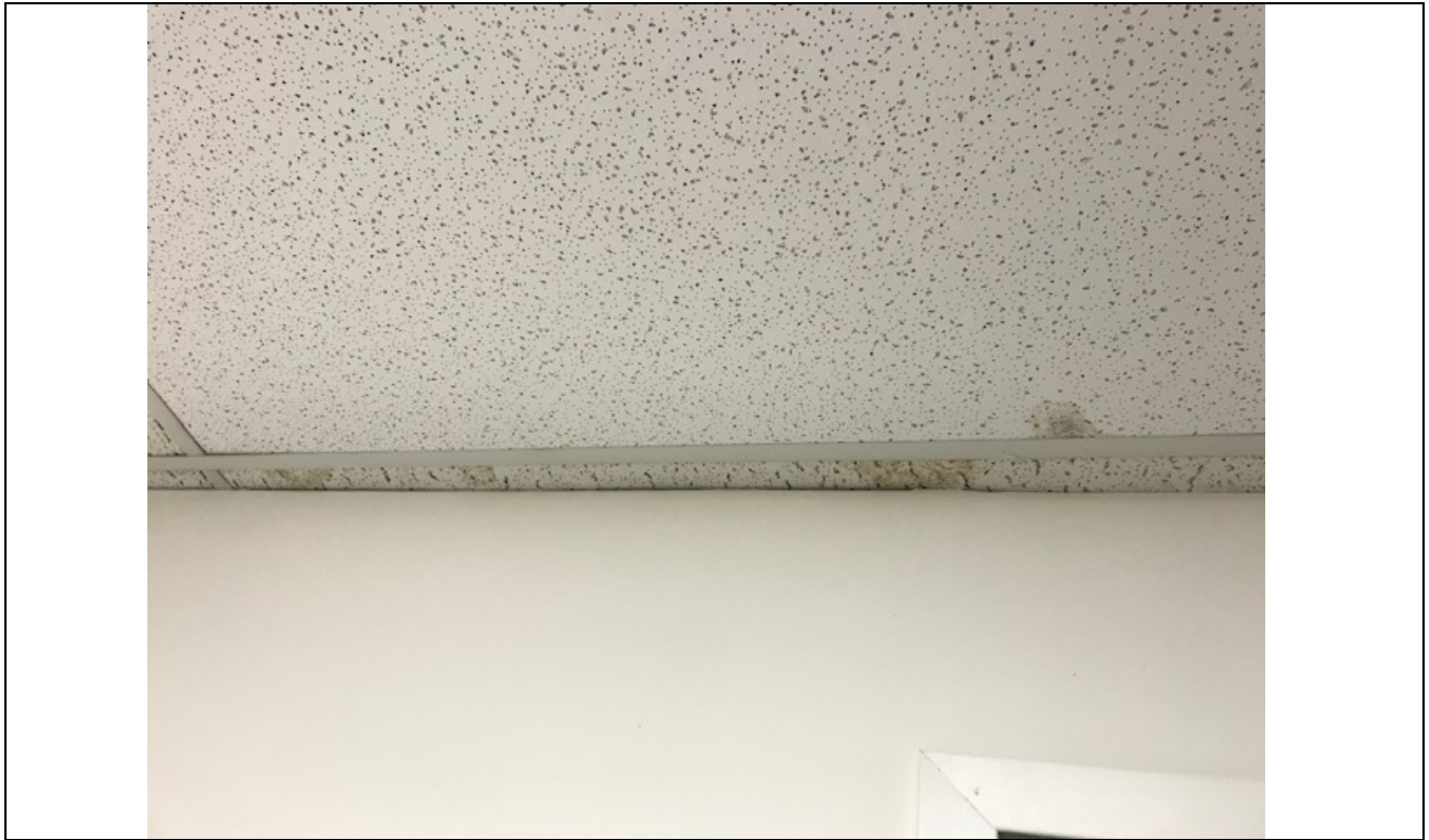
Photo No. 3: CB Building, Room 109 – Ceiling tile with minor water stains.
