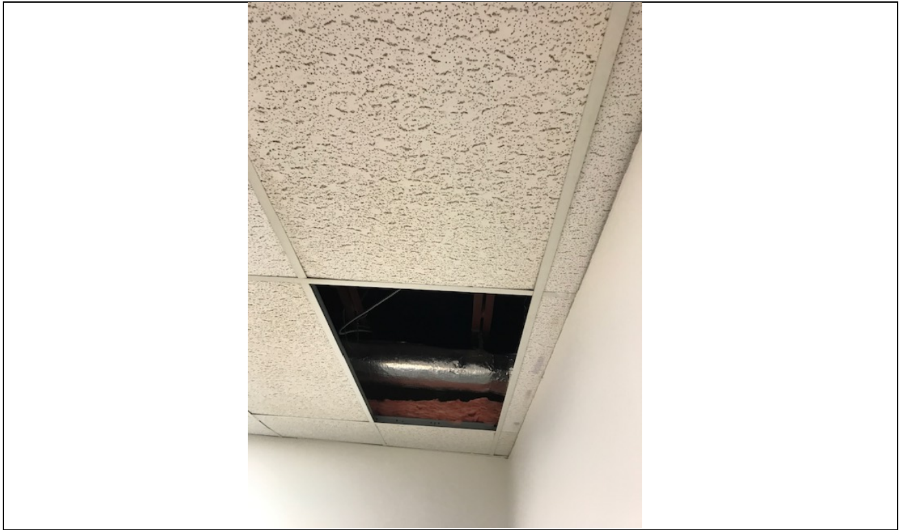
Photo No. 5: CB Building, Room 116-H - Missing Ceiling Tile.
